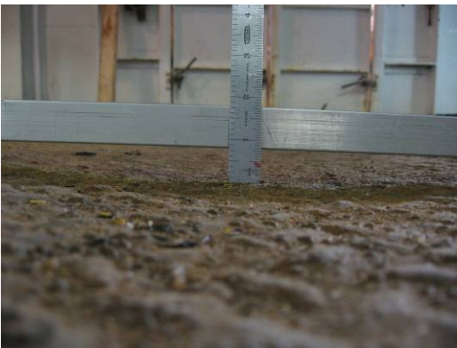
Buckled down – 13/16” depth
