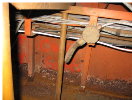
Corroded steel and coating failure
