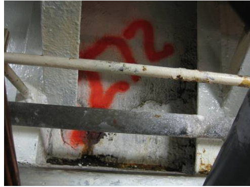
Corroded shell plating
