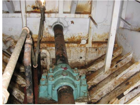
Coating failure and wasted frames
