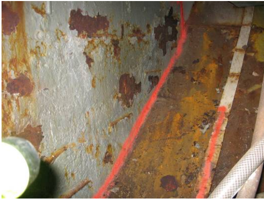
Bulkhead at frame #24 wasted
