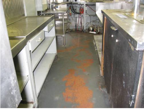
Worn deck in food service area
