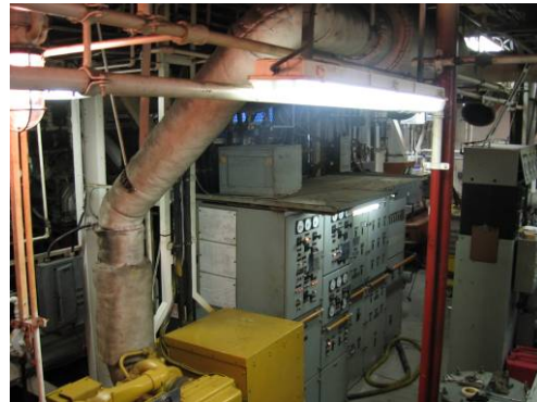
Main electrical distribution panels
