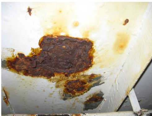
Deck wasted through in head at sink
