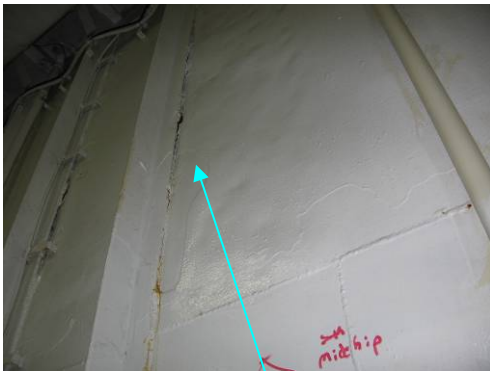
Cracked weld – buckled bulkhead
