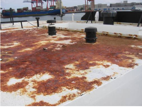
Housetop coating failure and active corrosion
