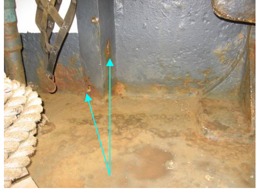
Superstructure with holes
