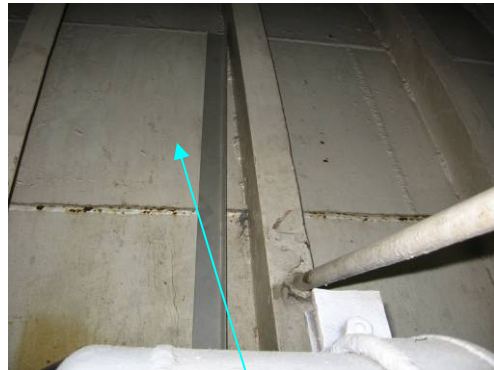
Plate inserted from previous bottom damage
