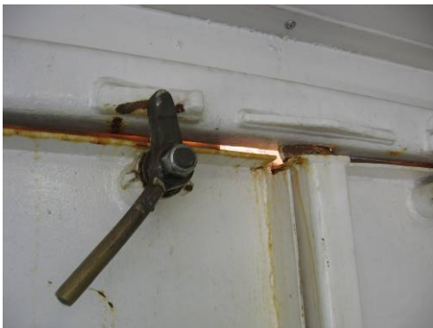
Watertight loading door will not close
