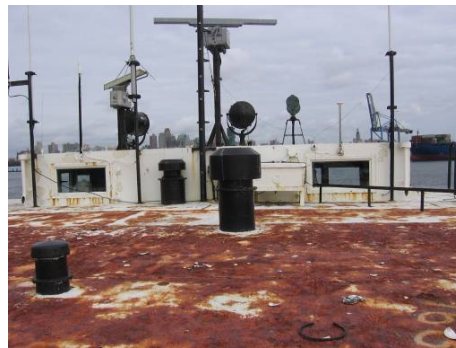
Antennas and searchlights and Housetop corrosion
