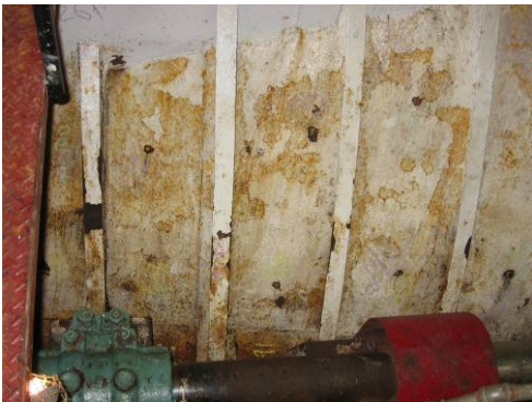
Coating failure – poor surface preparation
