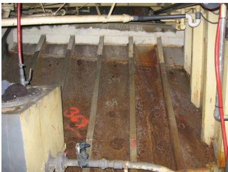
Coating Failure – active corrosion
