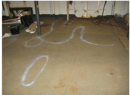
Outline – main deck buckled up
