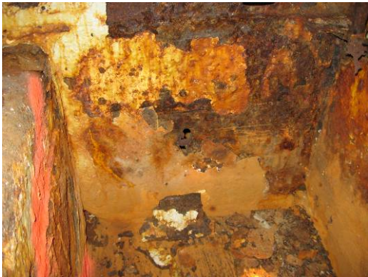
Holes in floors
