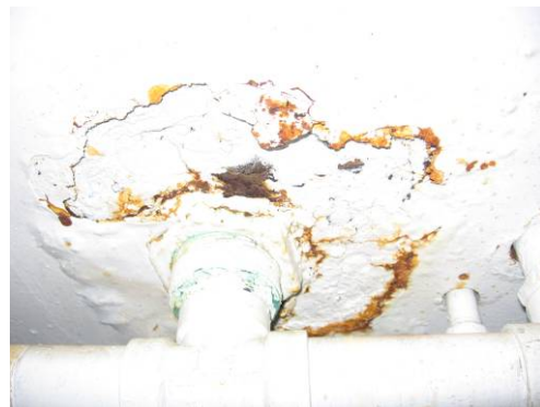
Deck wasted through at toilets
