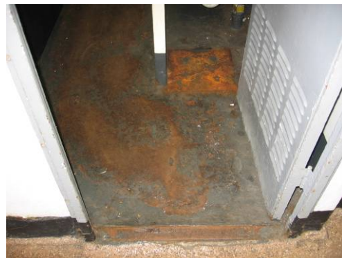
Wasted steel in salon deck
