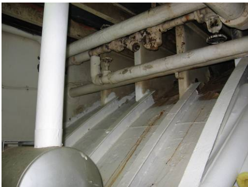
Coating failure in overhead
