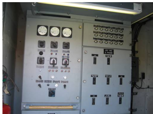
Emergency switch gear
