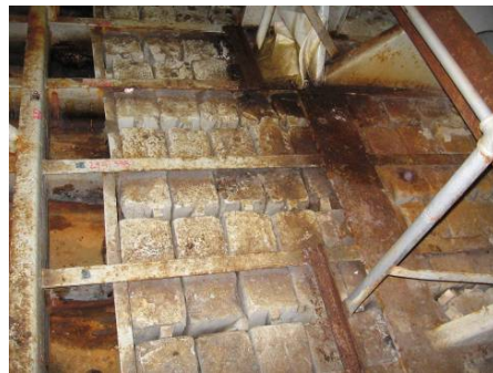
Lead ballast blocks
