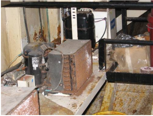
Corroded refrigeration compressors
