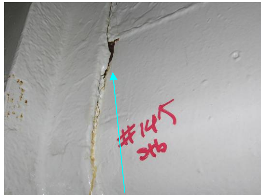
Cracked weld at frame
