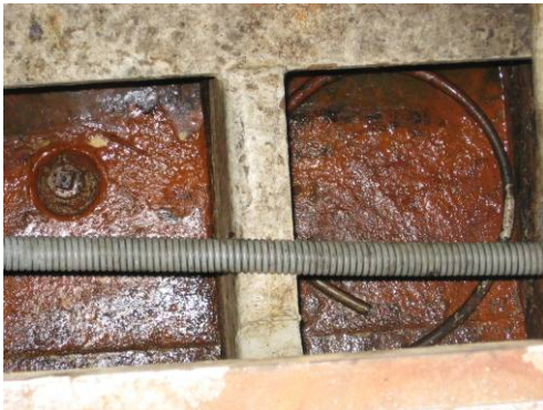
Corroded bottom plates
