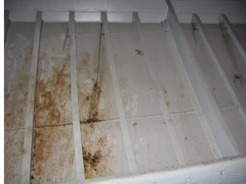
Localized coating failure
