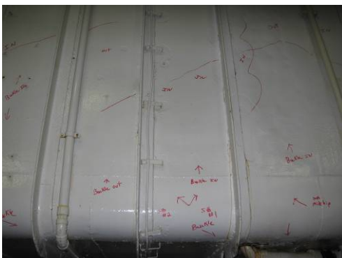
Buckled bulkhead - starboard midship
