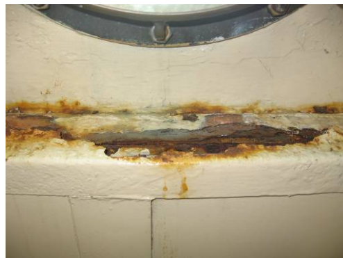
Corroded steel under porthole
