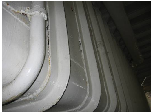
More cracked welds
