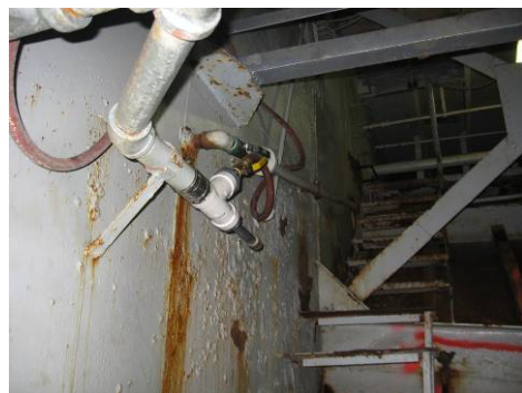
Wasted and buckled bulkhead #24 aft
