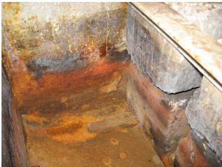
Wasted bottom plate next to lead ballast
