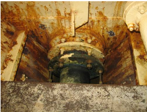
Wasted Steel bulkhead #47 aft
