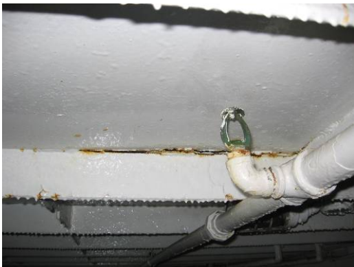
Cracked weld at deck
