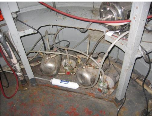
Galley service equipment
