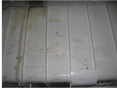
Buckled bulkhead - port midship
