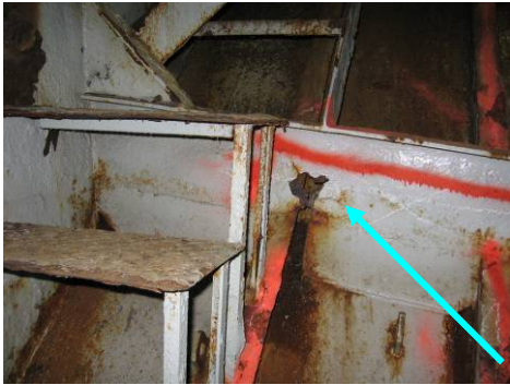
Hole in girder
