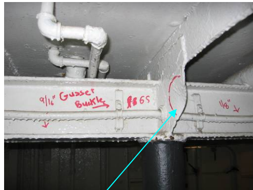
Example of buckled gusset
