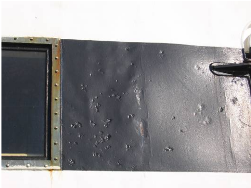
Pitting in superstructure
