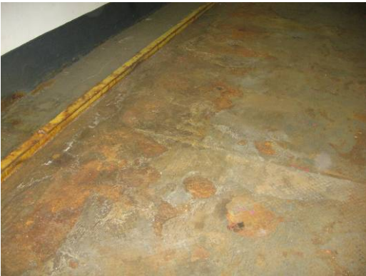
Significant coating failure
