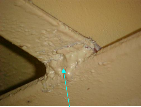
Crack in deck beam weld
