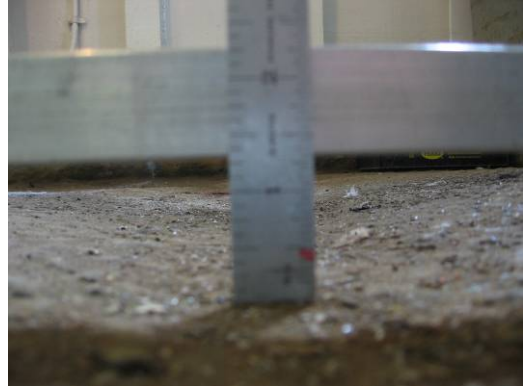
Buckled down – 1-3/8” depth
