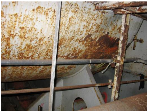
Corroded black water tank
