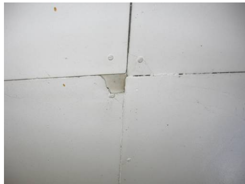
Asbestos ceiling in salon
