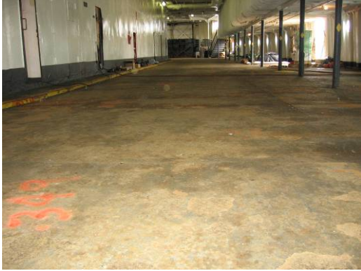
Wasted steel and coating failure
