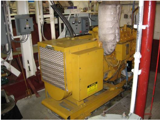
New AC Generator
