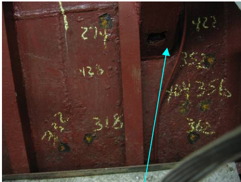
Hole in frame
