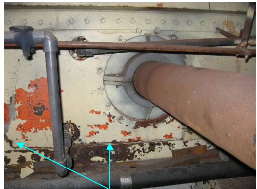
Failed Bulkhead gasket
