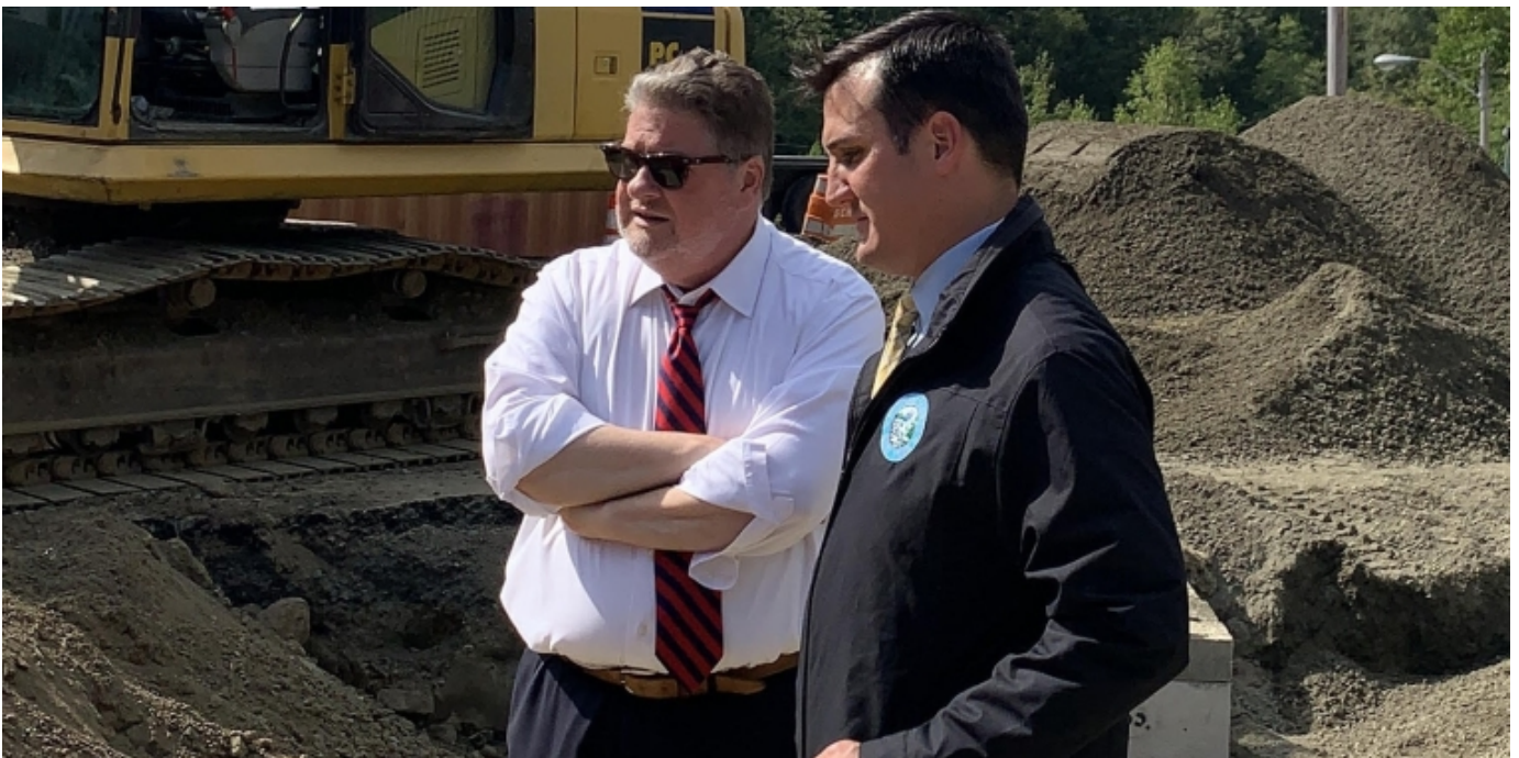
New York State Sen. Pete Harckham with Putnam County Executive Kevin Byrne at the site of the new Fire Training Center in Carmel Hamlet
