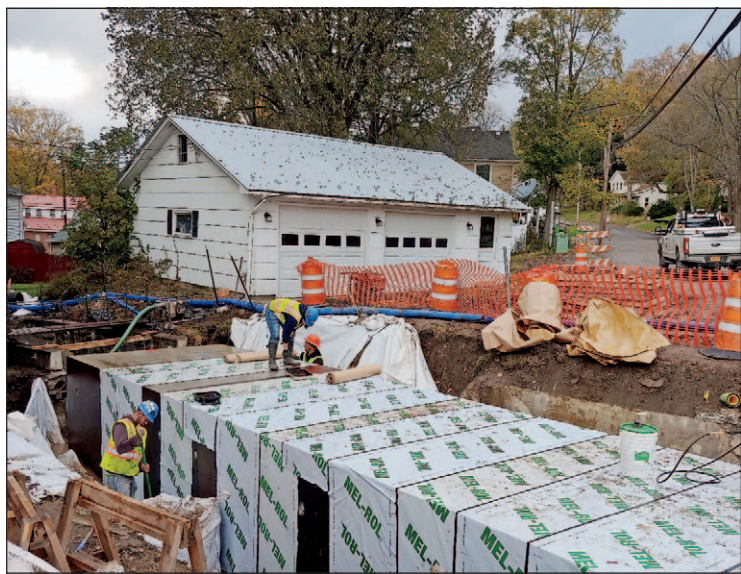
LC Whitford crews work on the Madison Creek box culvert project in the Village of Wellsville Tuesday. [CHRIS POTTER/THE SPECTATOR]
