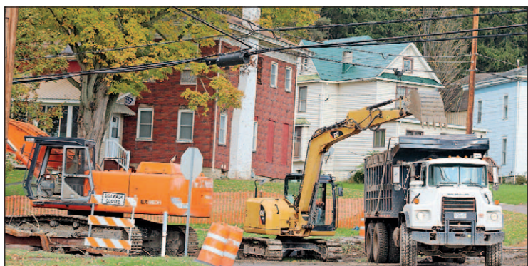
Earth is dug out for the Madison Creek box culvert project Tuesday in Wellsville.
