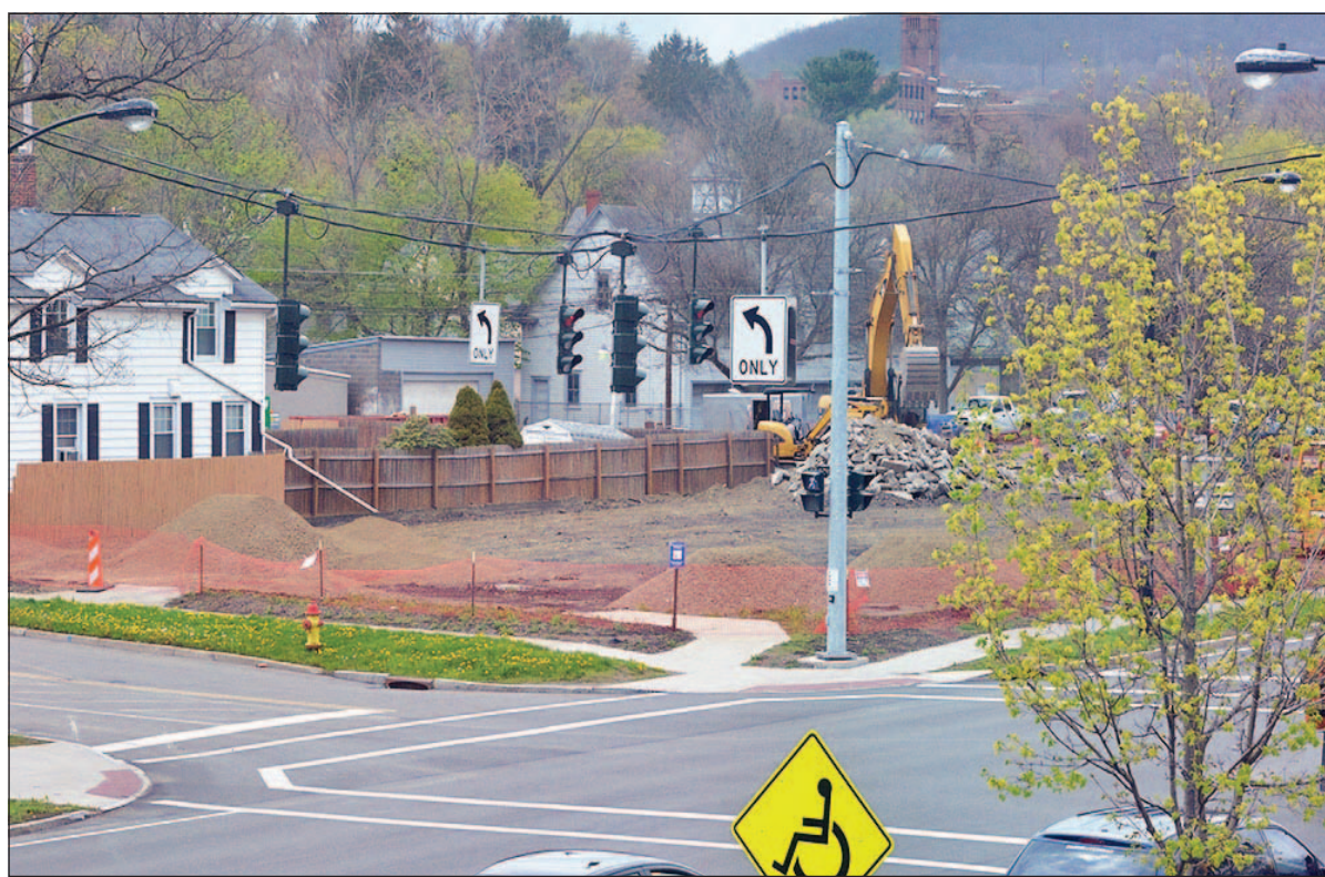
Site work is underway at the location of the future CCC Health and Education Complex on the corner of Denison Parkway and Chemung Street. ERIC WENSEL/THE LEADER
